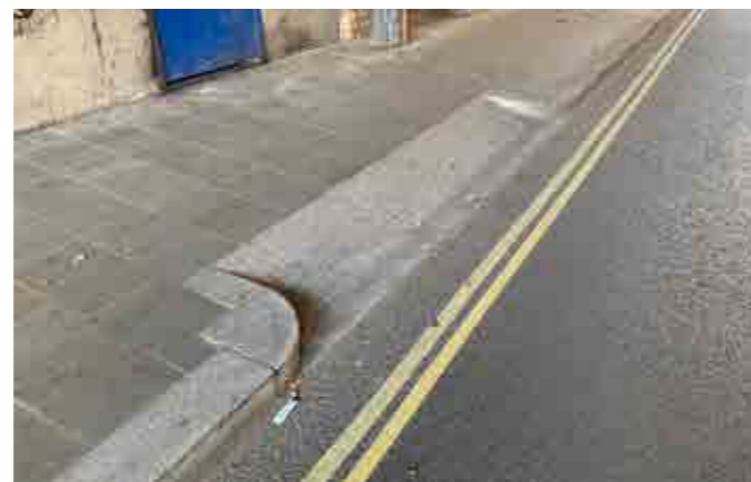
A good example of a footway crossover on Great Guildford Street on the Low Line, in this case for bin access.
