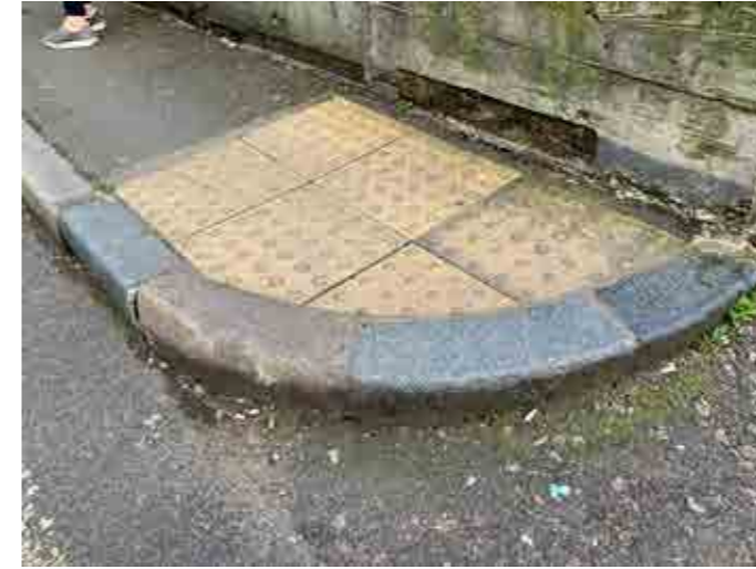
Poor quality footway surfaces + transitions
